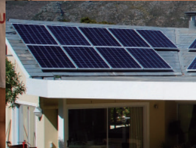
10KW | Cape Town, Güney A
